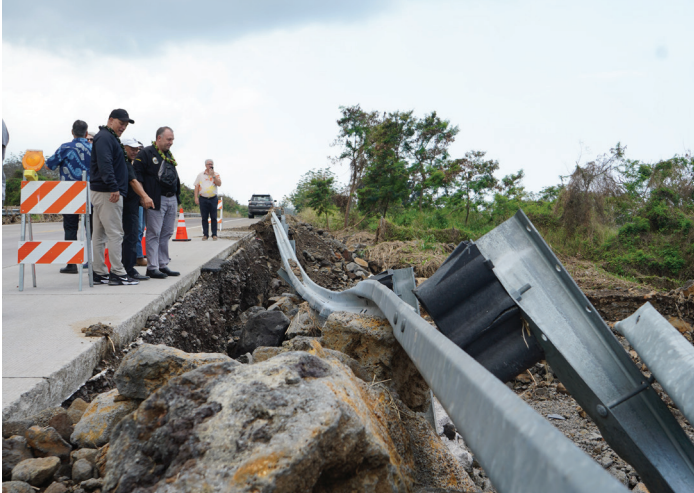
Governor Green, Hawai'i County Mayor Kimo Alameda and other officials tour the flood damage at Greenwell Farms.
